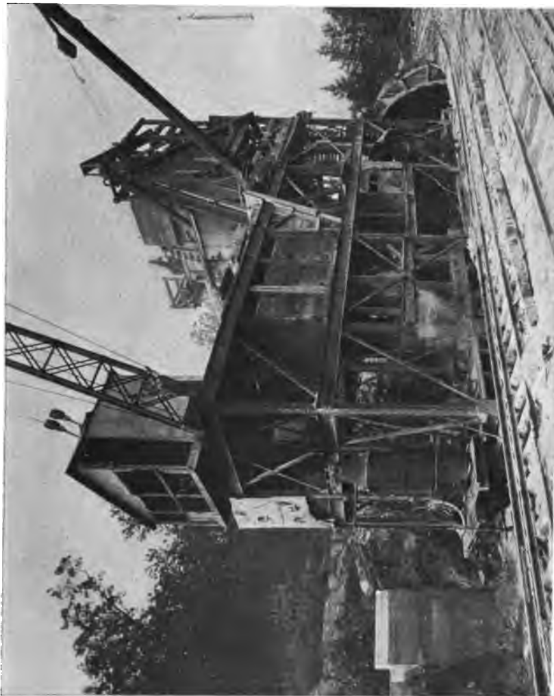
PLATE 66.—Contract 11. Body of Traveling, Crushing and Concrete Plant. Wooden Derrick was Air-driven and Raised Stone to Crusher. Steel Electric Derrick Raised Sand and Cement.
